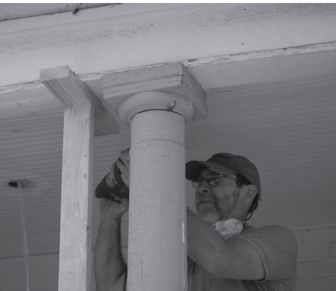
Michael Mahaffey of Home Tech, Inc. demonstrates wood repair on a column during the August Rehab it Right! Demonstration Workshop.
