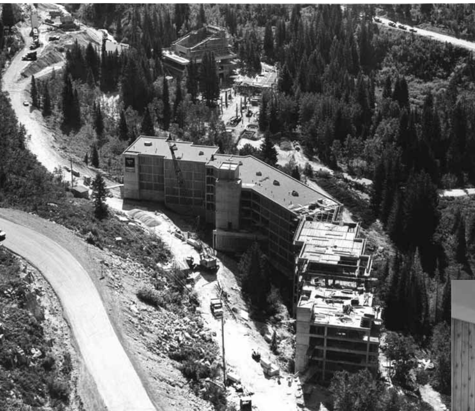
The photo above shows Snowbird with both the Lodge at Snowbird and the Tram Building in the later stages of construction,
