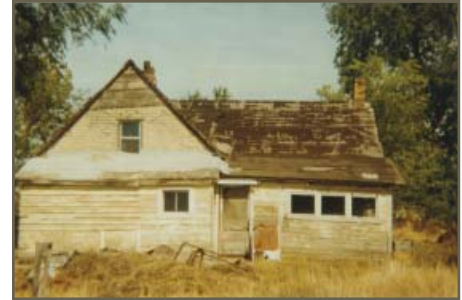
Spring City home before rehabilitation
